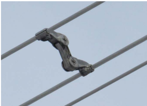
Spacer damper installed on transmission line
