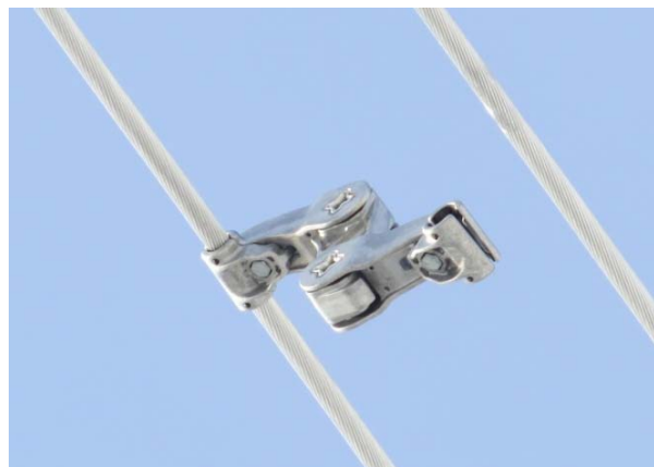
Spacer damper in a failed position
