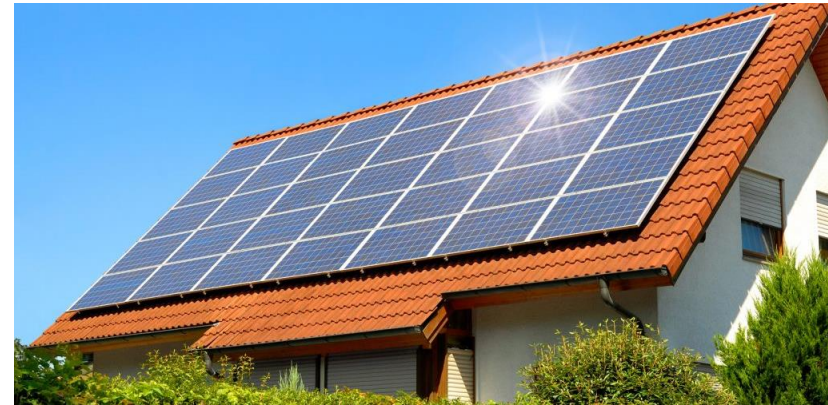
Source: Mays Building Services
